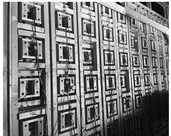
Backside view of Porcelain Membrane Wall . Photo: Adi Hollander.
